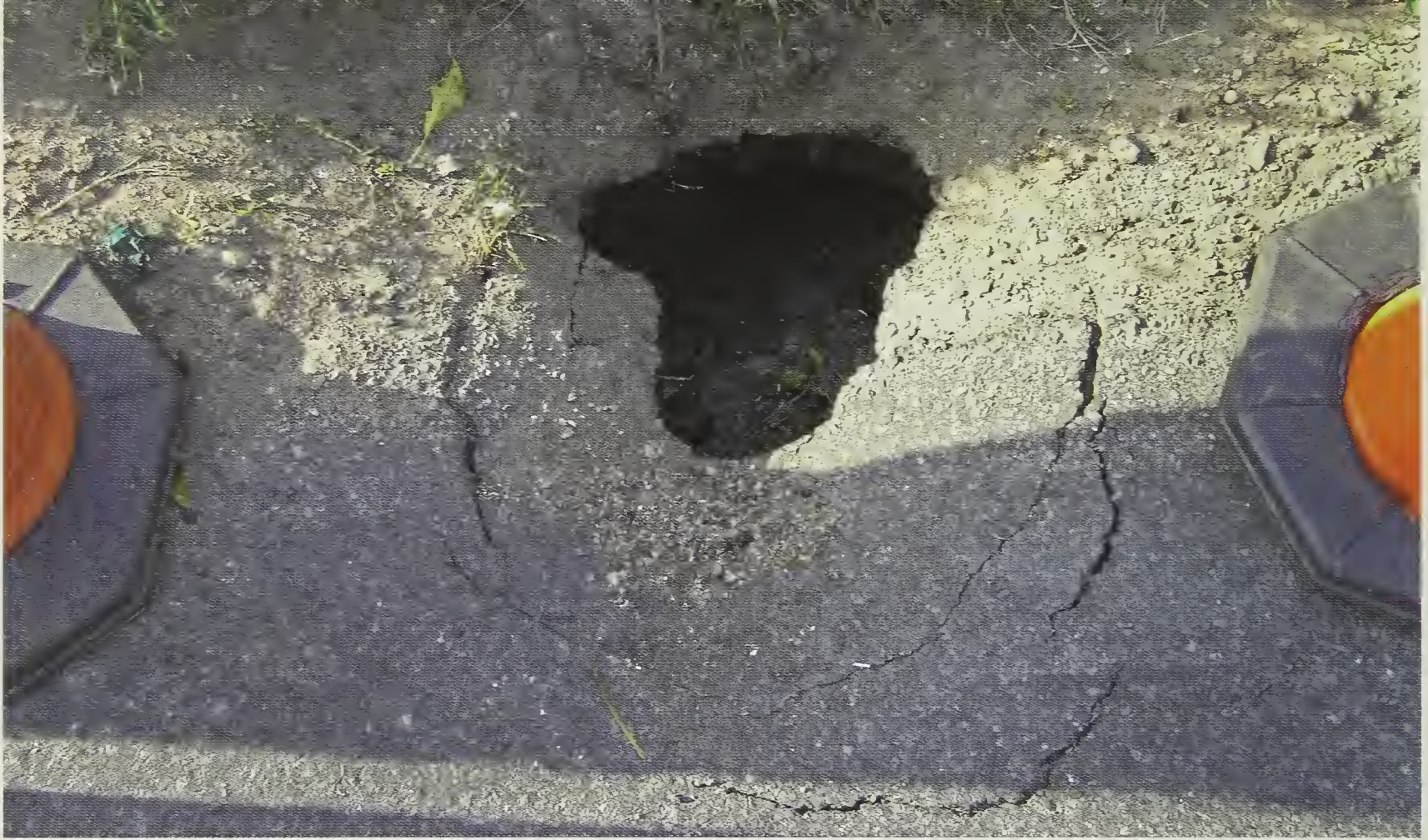
Badger damage to a Norfolk Road Badgers are powerful diggers and in some circumstances can cause significant damage. See article. Photo: John Crouch.
